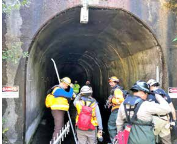
Spirit Lake Tunnel annual inspection team with engineers from Forest Service and U.S. Army Corps of Engineers, and a confined rescue team. Photo courtesy of USDA Forest Service Pacific Northwest Region
