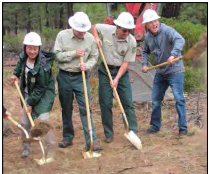
On October 20, 2014, Robin Gyorgyfalvy, District Ranger Kevin Larkin, Forest Supervisor John Allen, and Matt Freeman of CS Construction broke ground for the Cascade Lakes Welcome Station.
