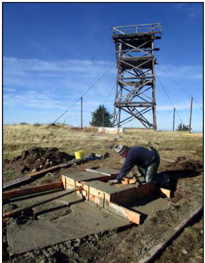
The historic Wildhorse Lookout tower structure loomed above the outhouse project on Saturday, October 18, 2014.
